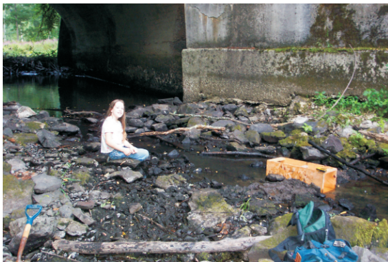
Temporarily “gardening” the stream to get all the flow through the wooden flume
